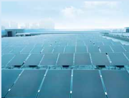
Rooftop solar power system at the plant in Henan, PRC
